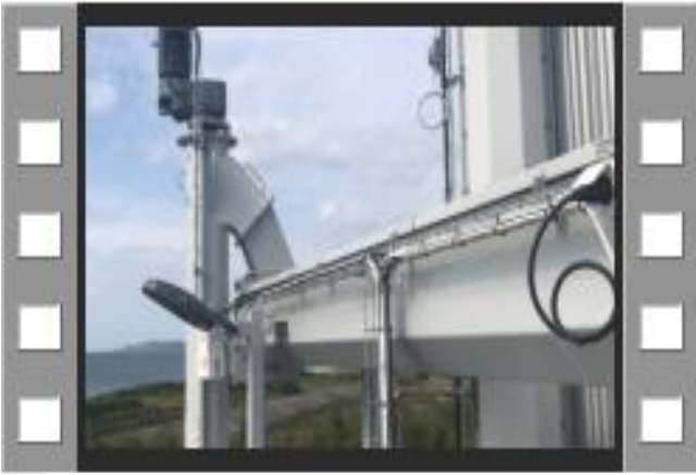
Test of the char transport system without material.
