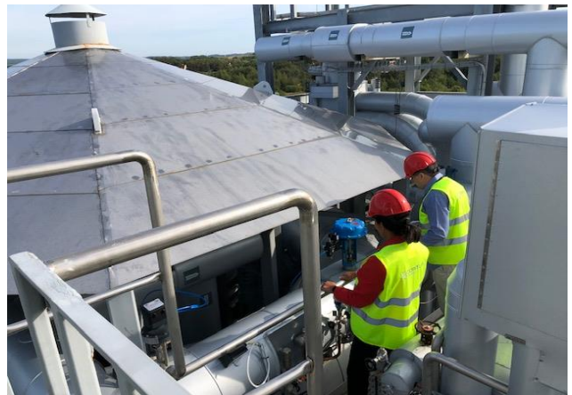
Cortus Martina Montesino Malmberg together with Jörgen Held from Renewtec at the top of the gasifier.
