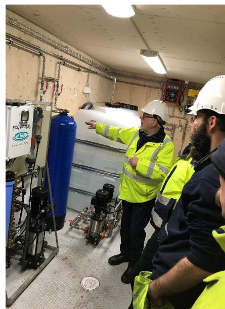
Education of the water purification system by our supplier, Pannpartner
