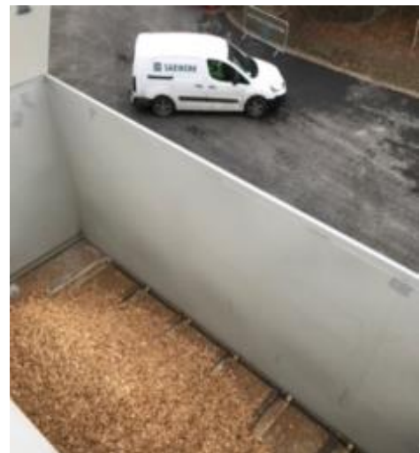
The biomass pocket contains 80 m 3 and is the starting point of the WoodRoll® process which after several steps converts biomass to an energy-rich synthetic gas with a high content of hydrogen.
